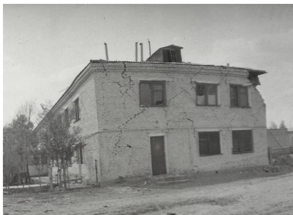
Pic. 2. The damage in a two storey brick building
